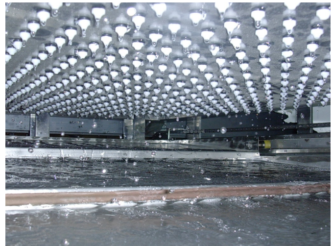
Fig. 5. Detail of the rain enabling / disabling system.
